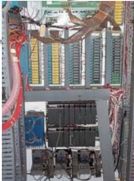
Typical panel at Grand Canyon handles between 100 and 250 Ethernet-based I/O.
