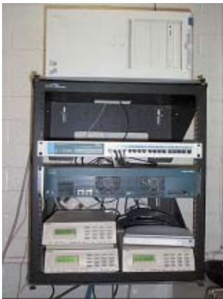
At the Grand Canyon site, interconnecting technologies spread spectrum radio communications to connect the control.
