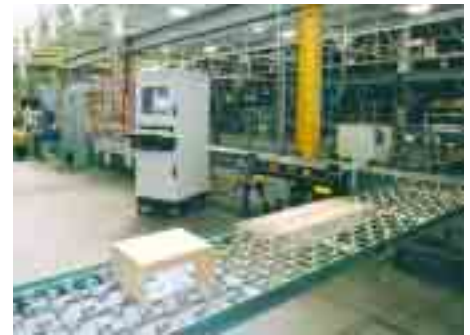
FloStor's material handling installation at Peet's Coffee & Tea (control station at center)
