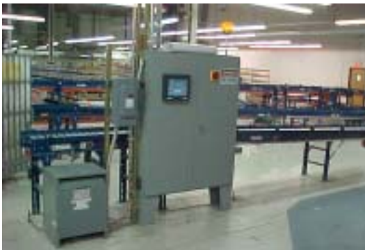
Control panel with HMI and motor starters at conveyor’s end.
