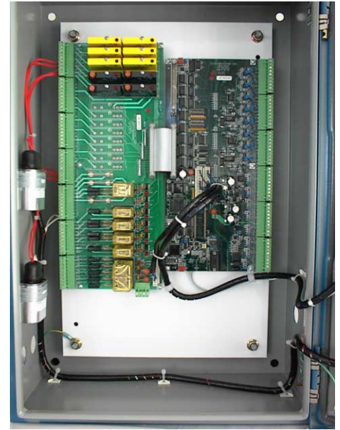
Intelligent Analog Module in the main panel has a ModBus interface to the embedded controller with Think & Do
